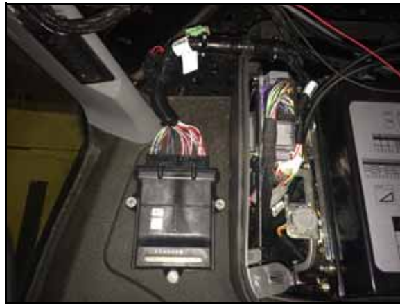
FIGURE 5. Node Harness Installed on SmarTrax Node
