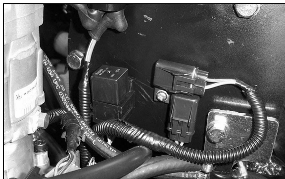
Located rear side of valve mounting bracket.
