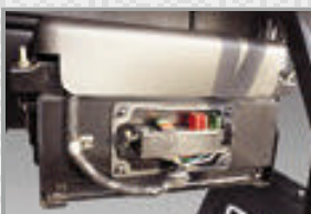
Auxiliary fuse box
