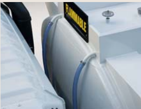
Drain Pipe & Hose
