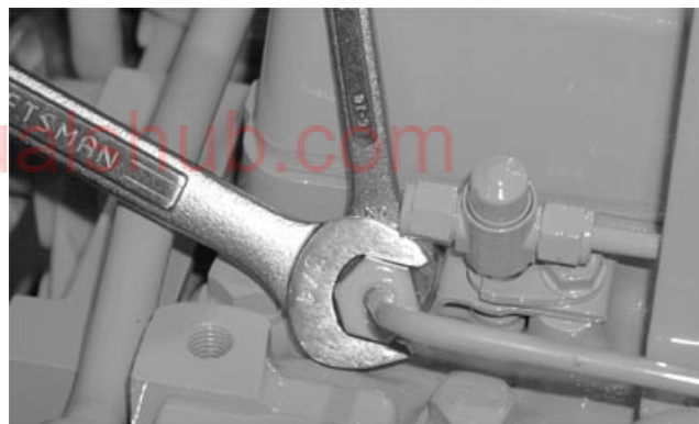
Nozzle Fuel Pressure Line
