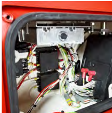
Electric cabinet is easily accessible.
