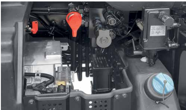
Circuit 2 hydraulic valve block
