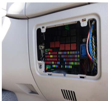
Figure 7-2.2 Inside View - Electrical Junction Box Location
