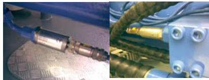
Pressure transducer installation
